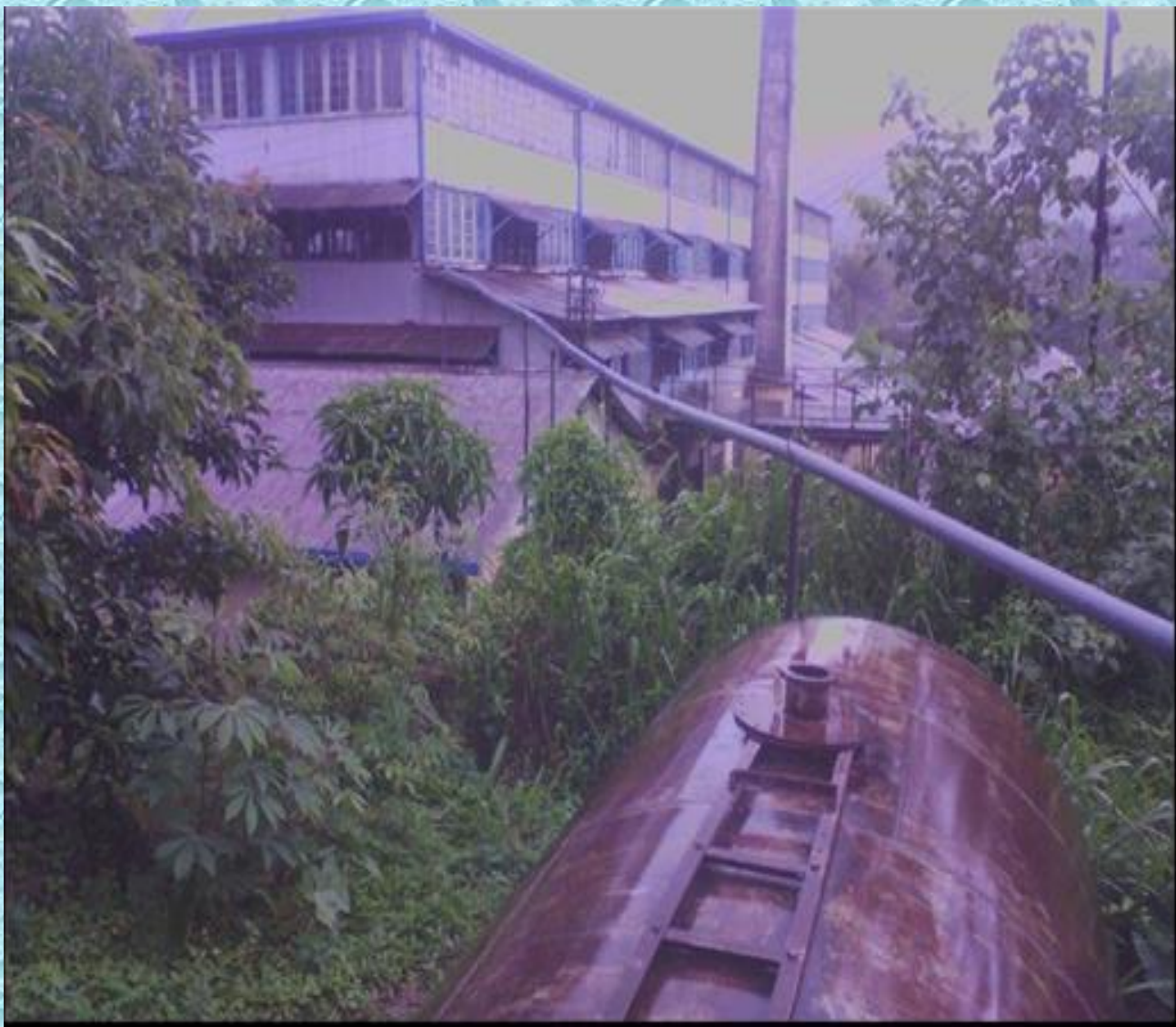
Roof rainwater harvesting at Meddecombra tea factory
